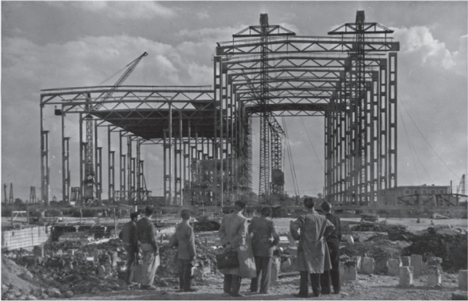
■ Illustration 5. Tiszapalkonya power plant 1952-57, Gy. Mátrai, K. Pászti, lifting the trussed main girder
