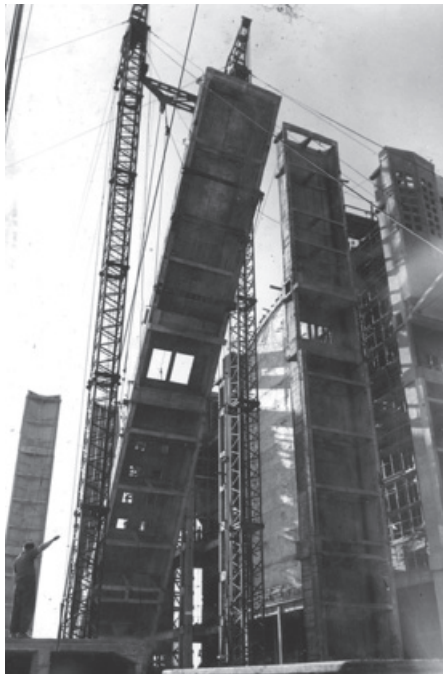
■ Illustration 7. Pécsújhely power plant 1955-59, Gy. Mátrai, K. Pászti, lifting the cupboard-like spatial pillar between boiler house and turbine hall
