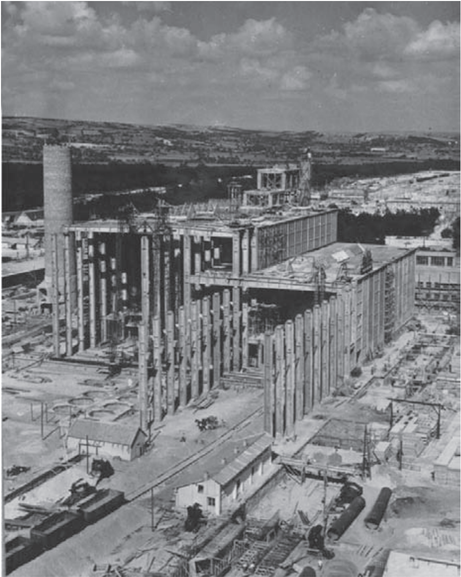
■ Illustration 2. Inota power plant “7 th November”, 1950, Gyula Mátrai, Károly Pászti, under construction
